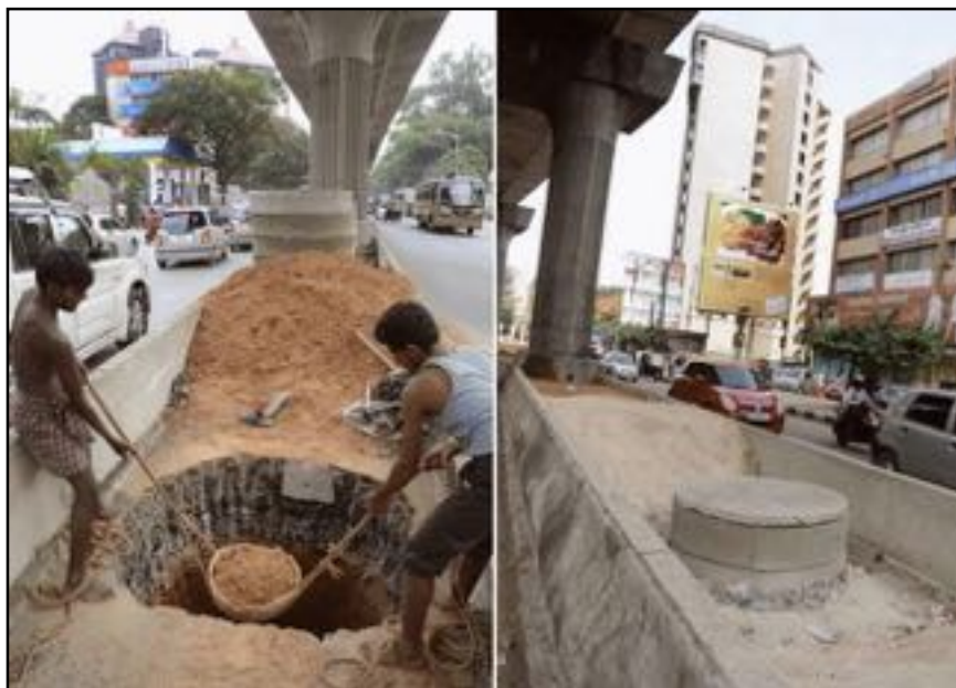
Figure 6-3: Rain Harvesting pits implemented by BMRCL along metro alignment
